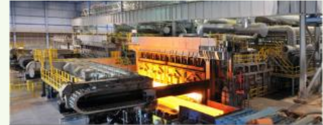
Walking Beam Furnace 300 tph Slab discharging temperature: 1250 °C Specific NG consumption: 1.3 GJ/ton
