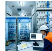
Automation, power and controls for the metals industry
